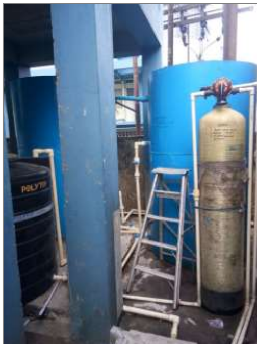
Effluent Treatment Plant 1
