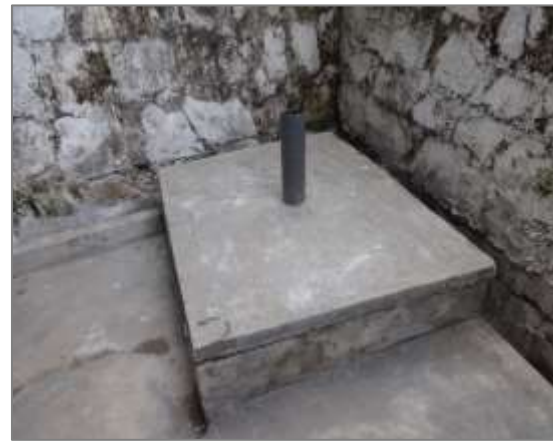
Underground Sharp Pit (needle disposal)
