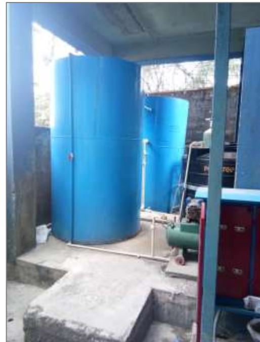
Effluent Treatment Plant 2
